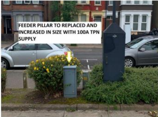
Feeder Pillar currently to be removed
